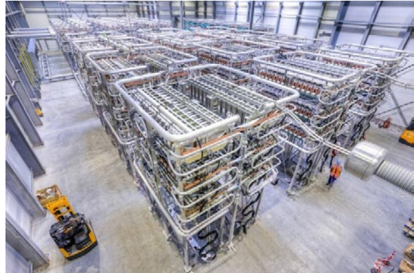
Figure 5: Interior view of a HVDC Plus converter station in Büttel in Schleswig-Holstein, the same technology as will be used for the COBRA converter stations.
