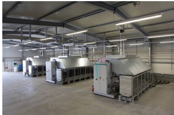
Figure 3: EnergiePark Mainz Siemens PEM water electrolysis
